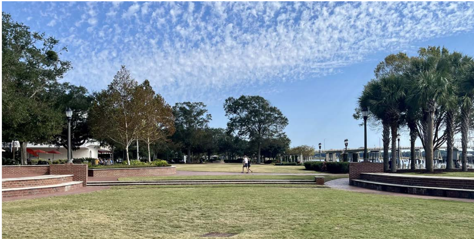
The relieving platform sits underneath the grassy expanse at Waterfront Park, and is in need of repair.
